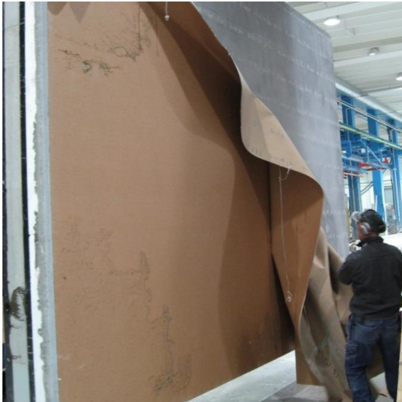
Once the concrete has hardened, it is removed from the mold and the paper is removed.
